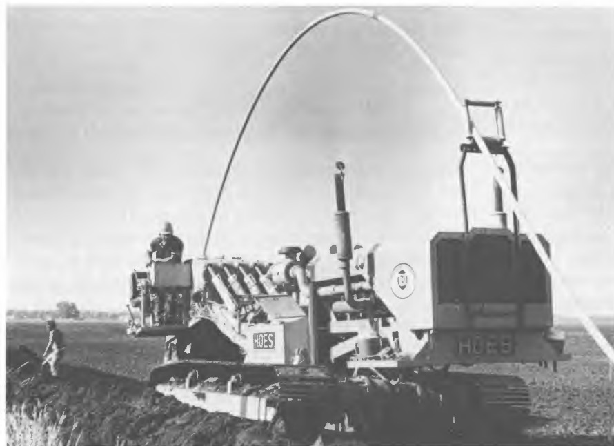
Fiber optic cable being buried near Oakland, Minnesota. The cable will connect at the Iowa border to become part of a transcontinental network, expected to be completed in the nineties.
